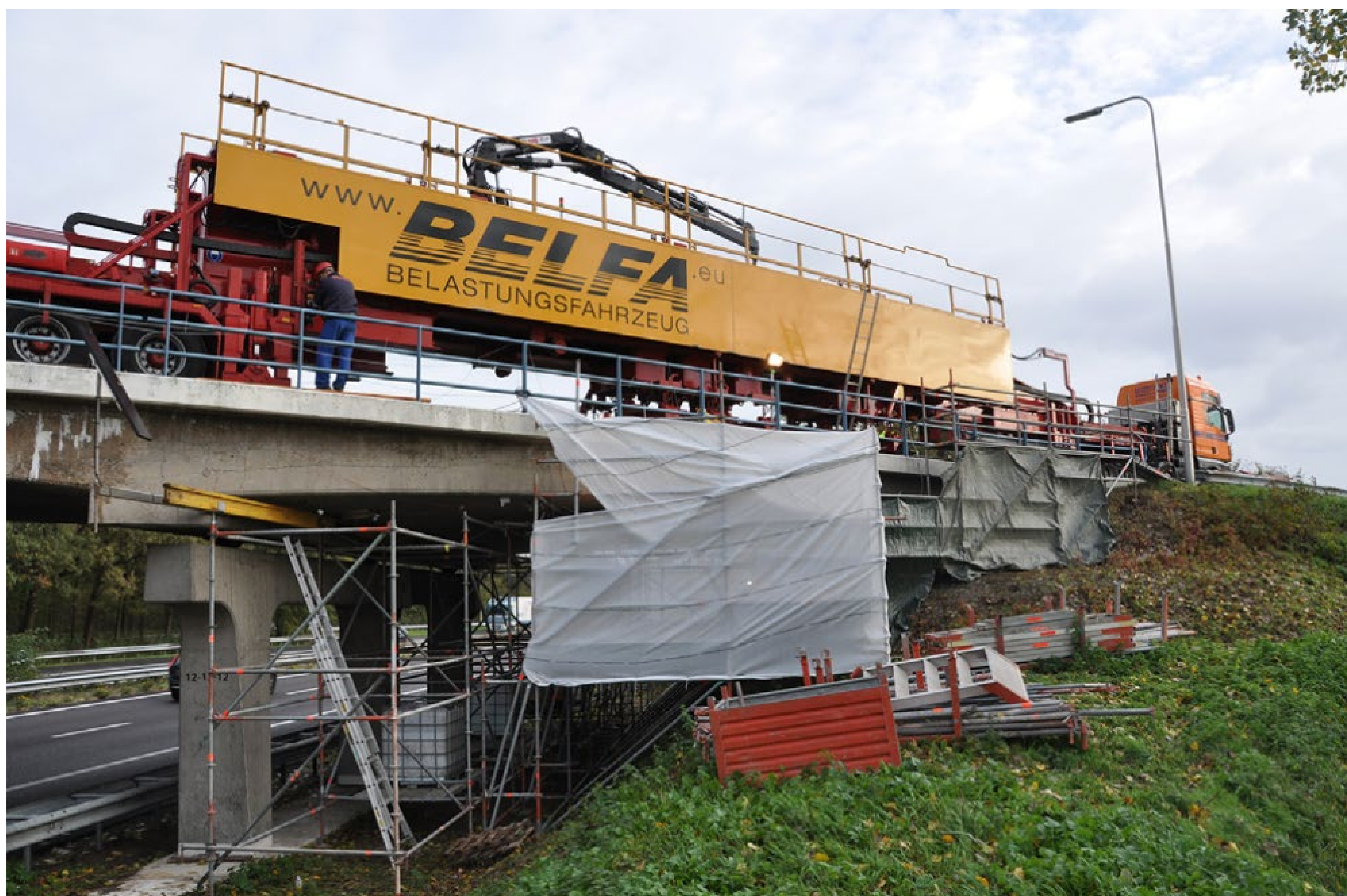
Pilot proof load test on viaduct Vlijmen-Oost using the specialized BELFA test vehicle
